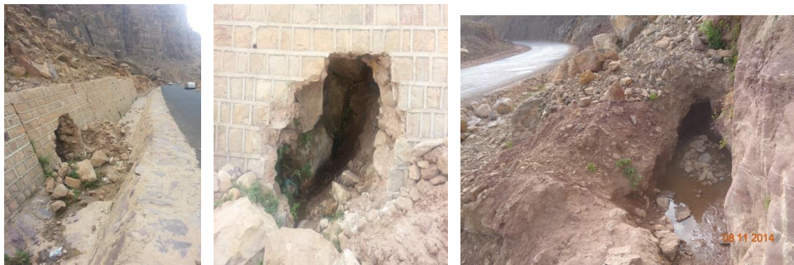
Figure 22. & 23. & 24. Neglecting spring source requirements lead to land users to dig the retaining wall (picture at the middle and left) to follow the spring flow which disappeared after the road construction and hill protection works. In other instances springs are re-excavated (picture on the right) after erosion
